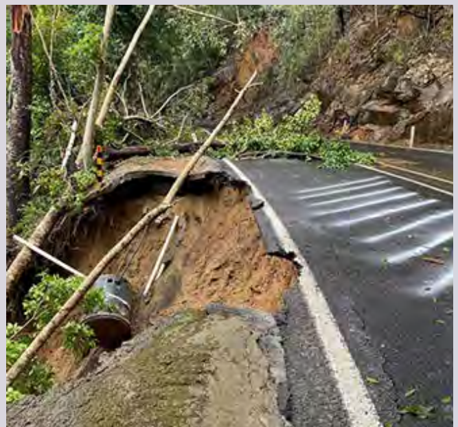
Kuranda Range Road – landslide
