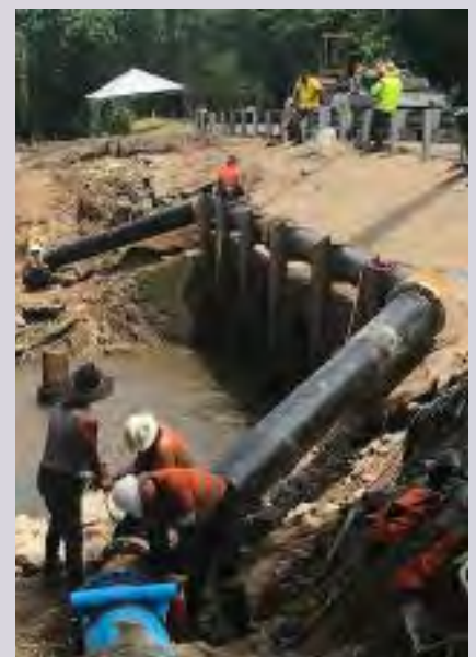
Image: Water supply outage as debris washes into treatment plant (courtesy: ABC News)
