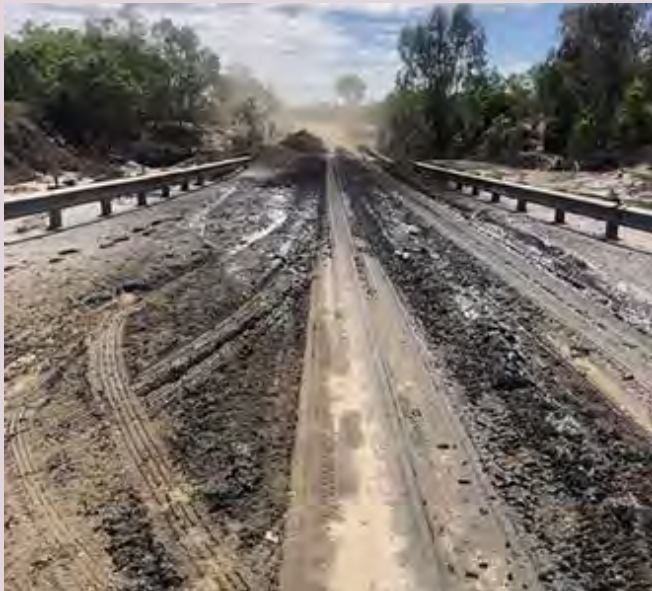
Mulligan Highway silt build-up
