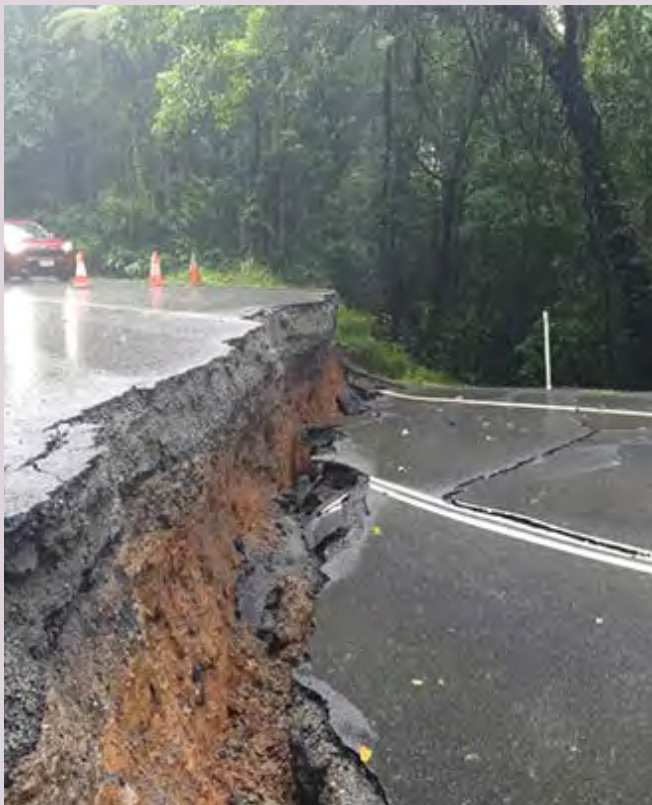
Image: Palmerston Highway major landslide
