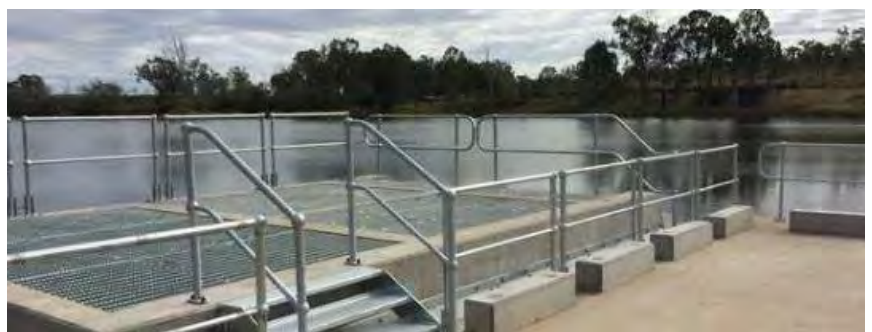
Image: Completed works on the Gayndah Water Supply Intake Station (courtesy: QRA)
