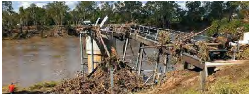
Image: Damage to the Gayndah Water supply intake station (courtesy: QRA)
