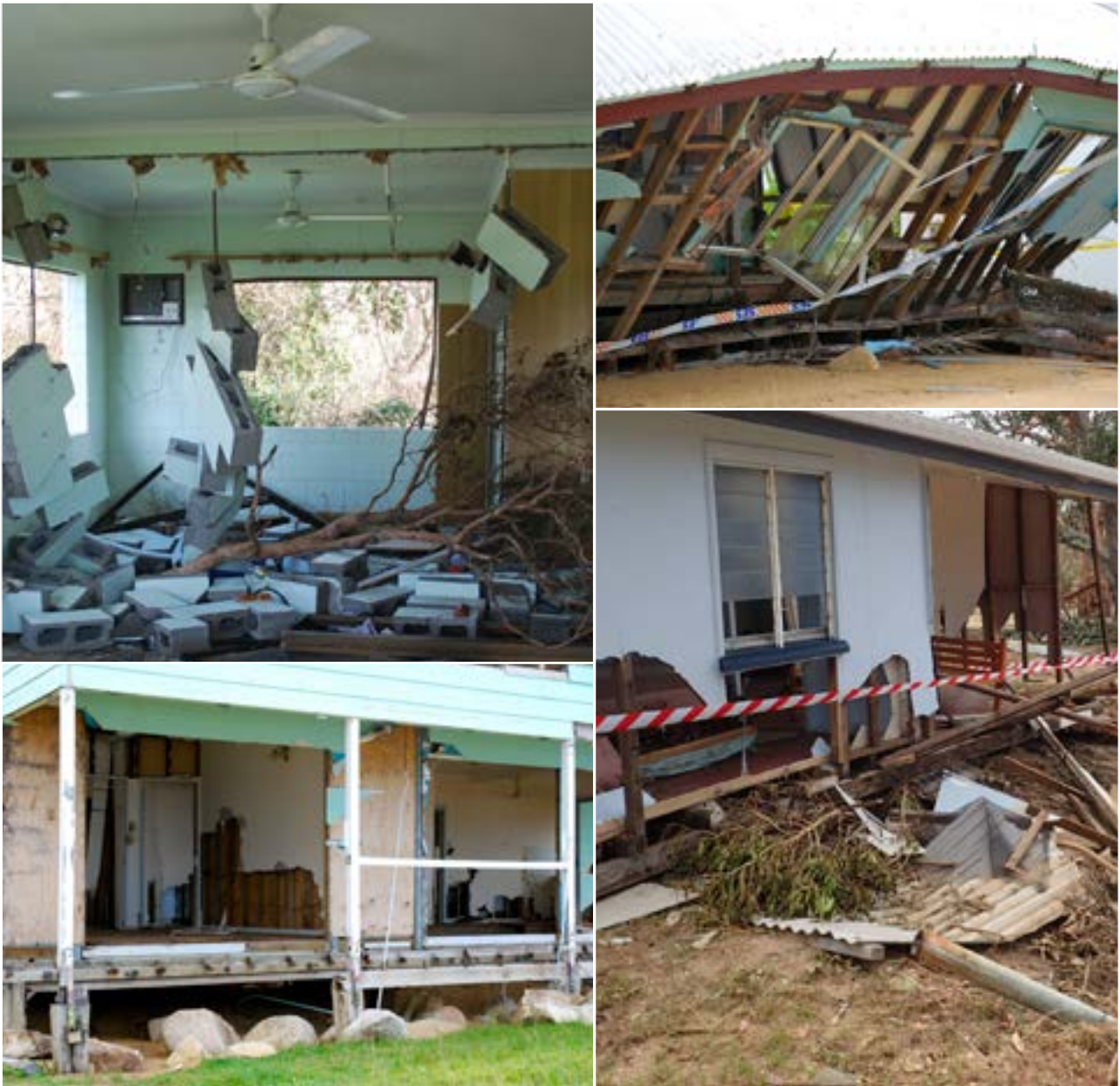
Damage to houses at beachside communities caused by storm tide inundation during Cyclone Yasi in 2011 and Cyclone Debbie in 2017. Some houses were battered by waters and pushed off their stumps, others remained in place despite extensive damage.
