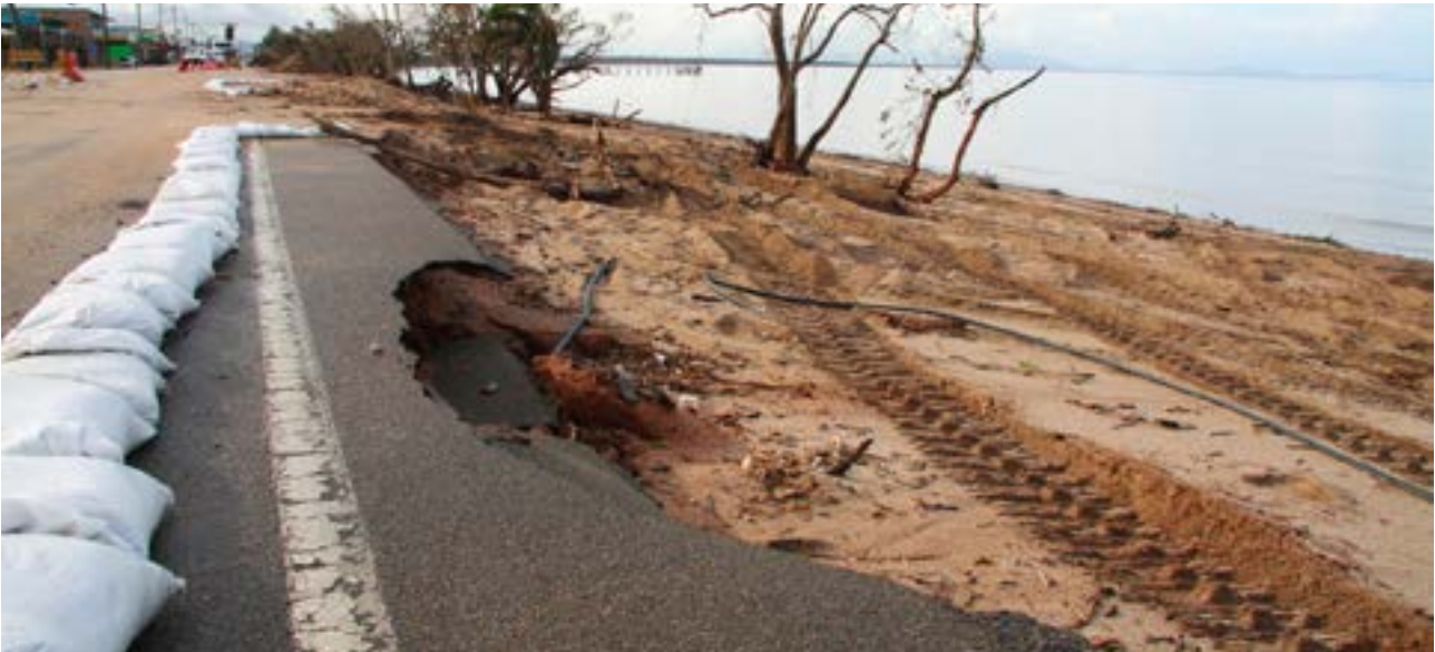
The storm surge from Cyclone Yasi ripped pieces out of the Bruce Highway at Cardwell, closing the northern artery for several days.
