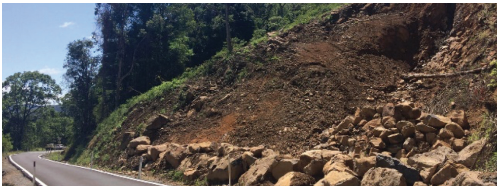
Nerang–Murwillumbah Road – landslip site
