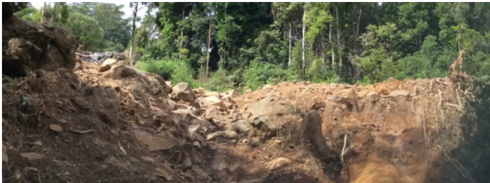
Nerang-Murwillumbah Road – landslip site
