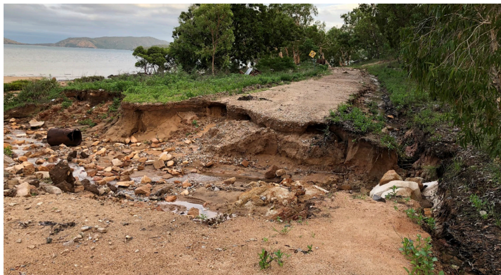
Road damage on Palm Island
