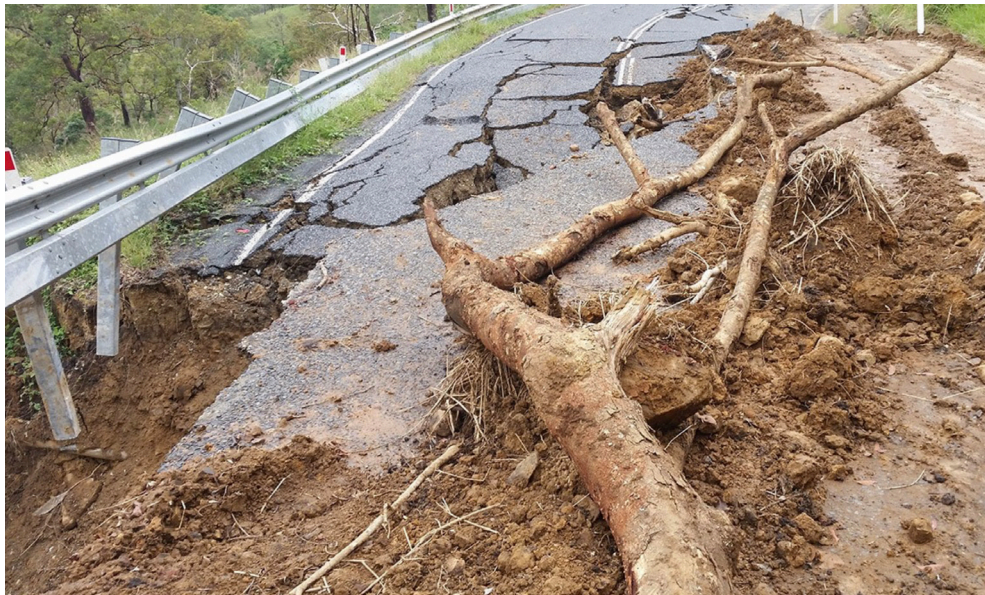
Marlborough-Sarina Road – damage at main slip site
