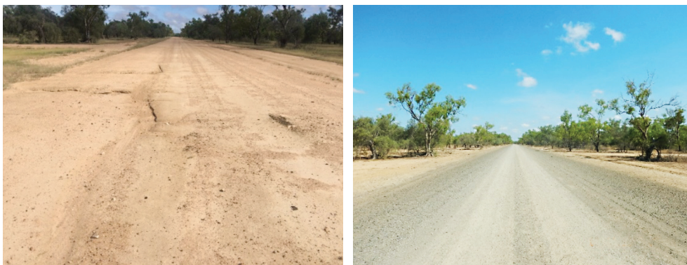
Dunbar to Kowanyama Road, Carpentaria Shire Council damage in 2016 (left) and post reconstruction (right)
