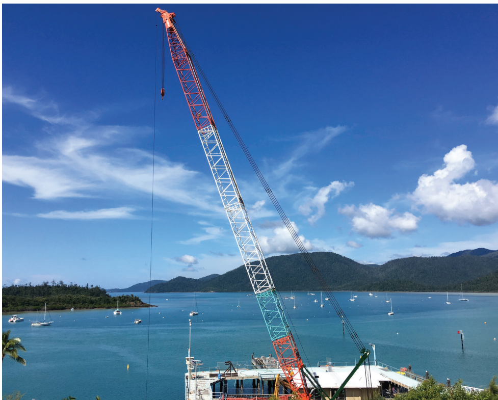
Demolition works underway at Shute Harbour (photo courtesy of Whitsunday Regional Council)
