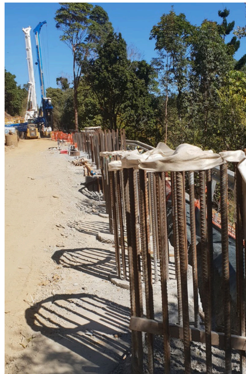
Nerang–Murwillumbah Road – finished piles prepared for construction of a concrete capping beam at the major landslip
