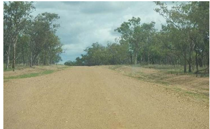
Gregory Developmental Road - damage caused by rainfall and flooding event in February 2014 (top) and following completion of reconstruction works (above)
