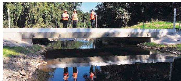
Derrier Bridge all but washed away in the 2013 events (top) and
