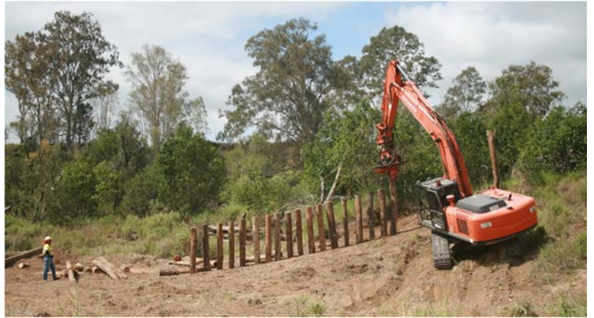
Start of restoration works – construction of the timber pile fields to further reduce velocity and support the establishment of new vegetation.
