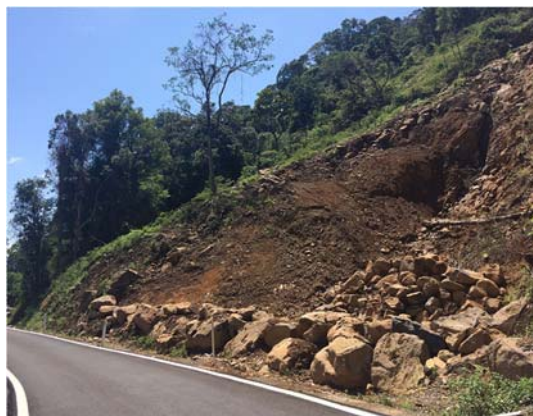
Above: Clean up of main landslide site on Nerang-Murwillumbah Road
