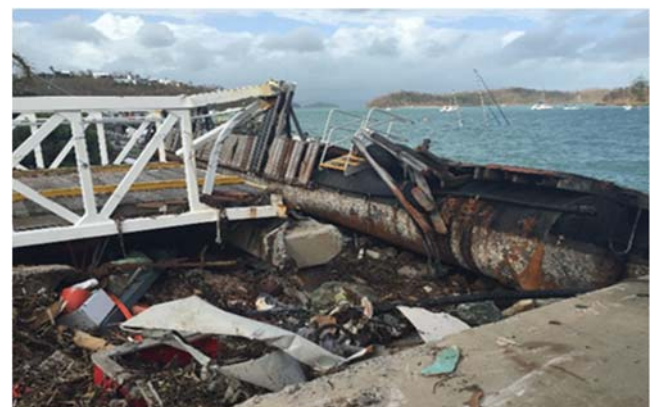
Above Shute Harbour in the Whitsundays suffered extensive damage.
