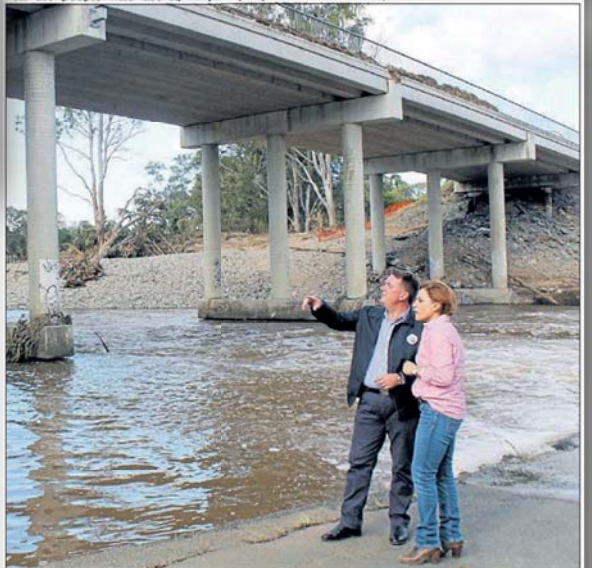
INFRASTRUCTURE FIX: Logan City mayor Luke Smith and deputy premier Jackie Trad inspecting the Alan Wilke Bridge in early April. Photo: Georgina Bayly
