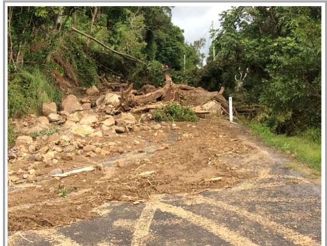
Image: Damage to State road assets by Severe Tropical Cyclone Debbie at Nerang-Murwillumbah Road.
