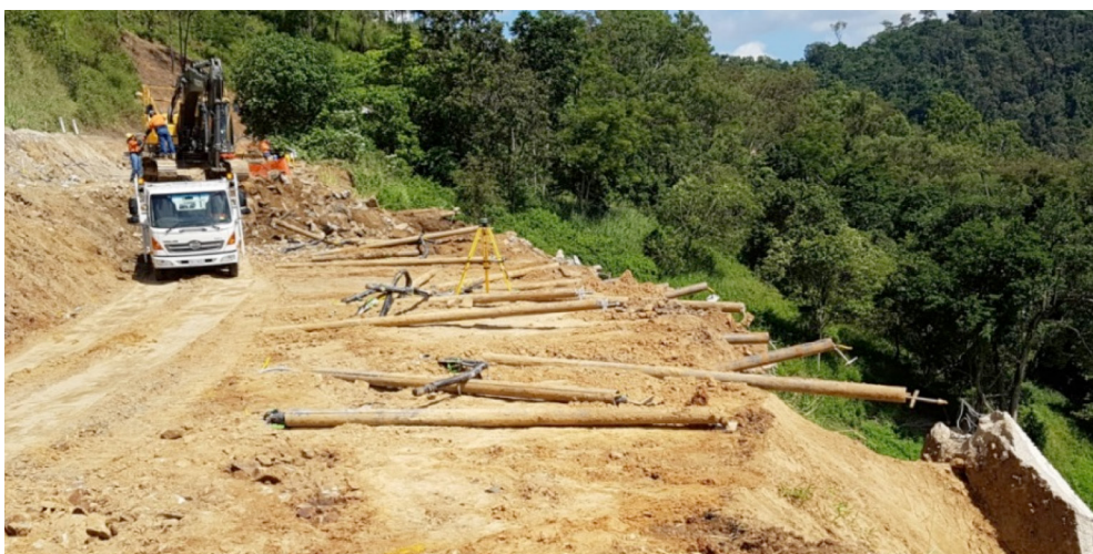
Sarina Range – excavation and placement of soil nails at main slip site
