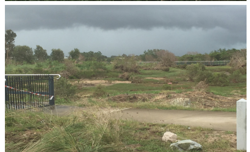
Damage to Mackay's Bluewater Trail and Queens Park following STC Debbie
