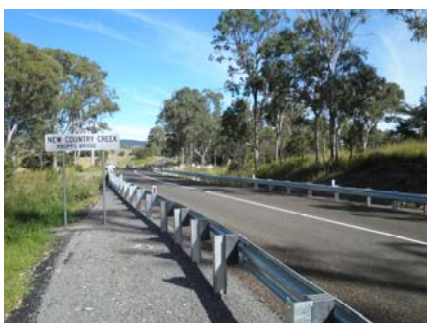
Left: Completed works at Kropps Bridge on Grigor Creek Road which was upgraded to a more flood resilient standard with Betterment funding
