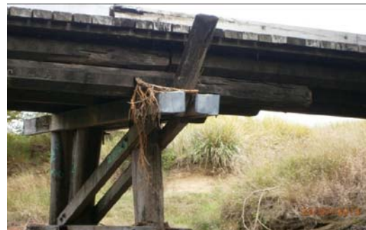
Damage to girders on Wunulla Lane Bridge from 2013 events
