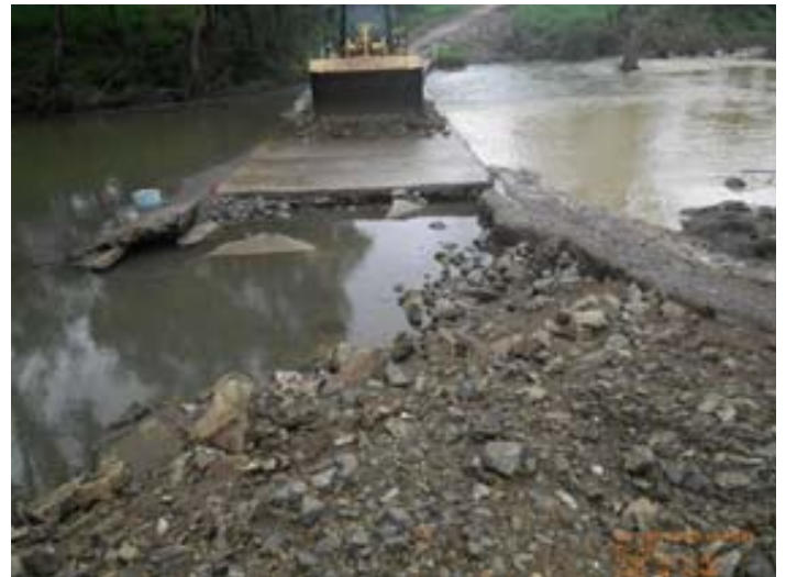
Upper Ulam Road damage post-Cyclone Oswald – January 2013
