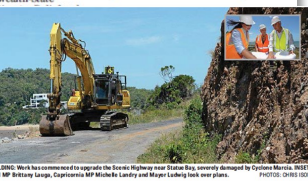
REOPENING: Work has commenced to upgrade the State Highway near Statue Bay, severely damaged by Cyclone Marcia. NEXT: Project MP Billie-Louise, Capricornia MP Michelle Landry and Mayor Ludwig look over plans. PHOTO: CHRIS DINE
