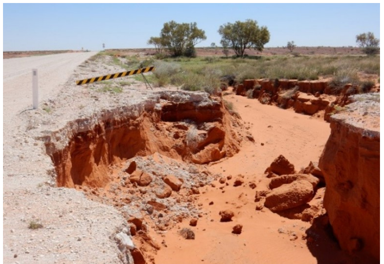
Birdsville Developmental Road – shoulder scour from Western Queensland Trough (March 2016)
