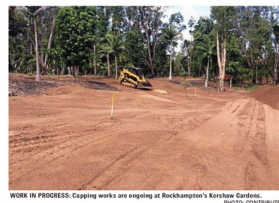
WORK IN PROGRESS: Capping works are ongoing at Rockhampton's Kershaw Gardens. PHOTO: CONTRIBUTED
