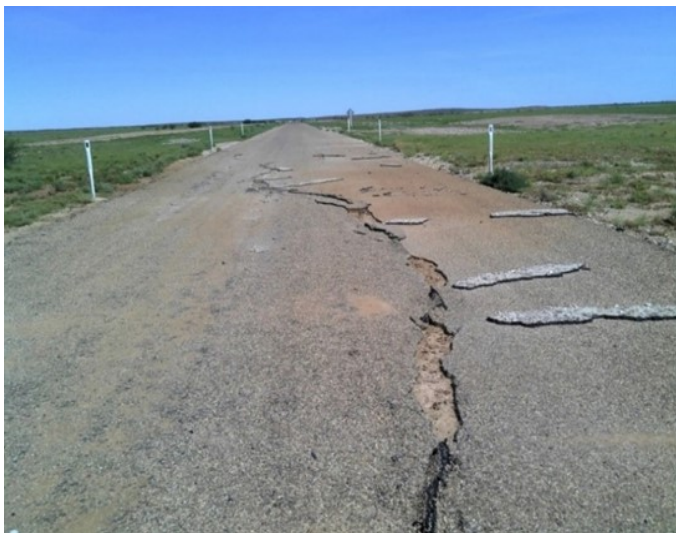
Diamantina Developmental Road (Windorah–Bedourie) – pavement seal damage from Western Queensland Trough (March 2016)
