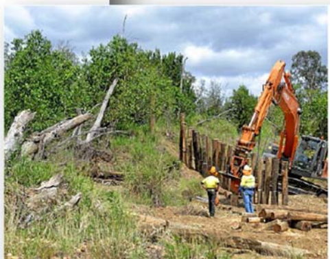
UNDER WAY: Pile fields under construction at the Sapling Pocket Inset Floodplain Restoration. PHOTO: ROB WILLIAMS
