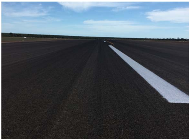
Works to repair the Normanton Airport runway included stabilising, resealing and additional line-marking
