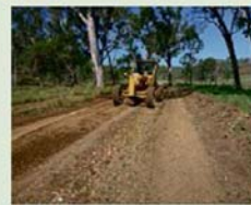
Goodys Rd, Monto 'under construction' Council acknowledges the Natural Disaster Relief and Recovery Arrangements (NDRRA) funding is a joint Commonwealth and State Government program.
