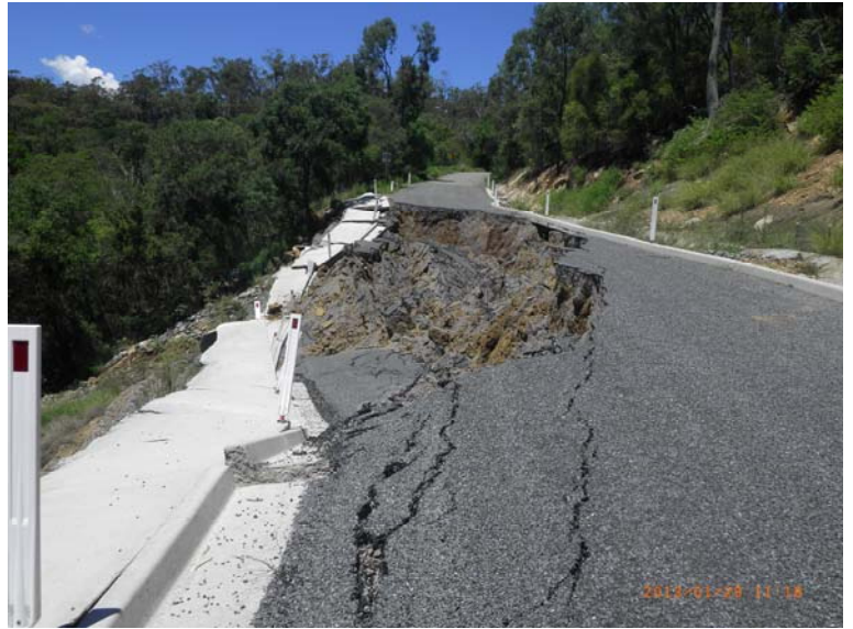
Major landslip damage to Flagstaff Road following the 2013 disaster events
