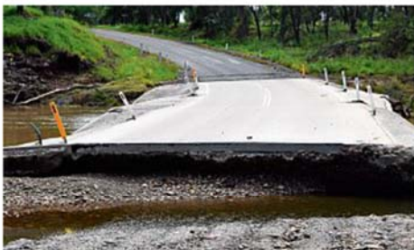
Callide Creek Crossing on Linkes Road after February's flood event.
