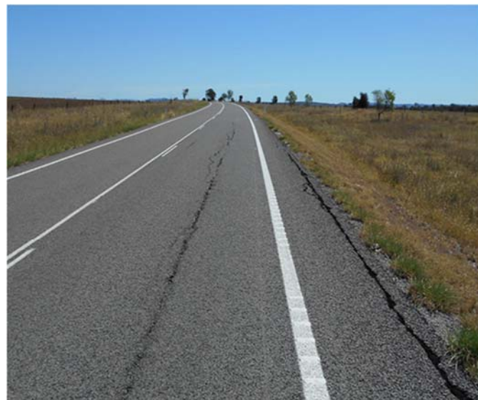
Leichhardt Highway (Westwood–Taroom) – damage to road shoulder and pavement
