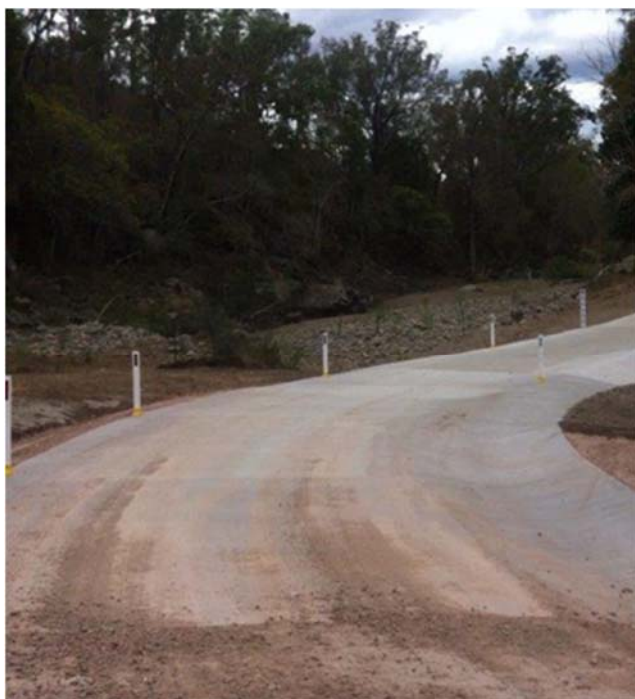
Damaged floodways on Rossmore Road following Tropical Cyclone Marcia (top and middle ) and following completion of betterment works (bottom)
