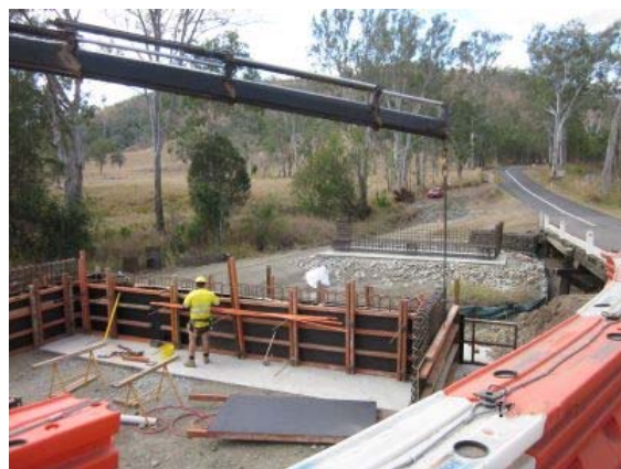
Council day labour crews undertaking works on replacement of Jones Bridge at Gregors Creek.
