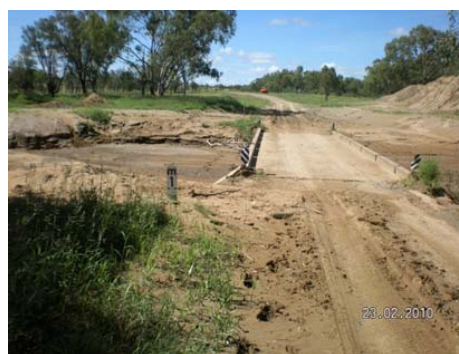
Left: examples of damage to sections of Portwine Road
