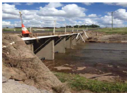
Undermined and fractured discharge aprons.
