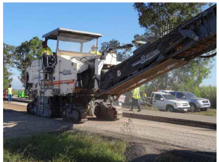
Above: Formation profiler, Bruce Highway (Bowen to Ayr) at Seymour River - October 2013
