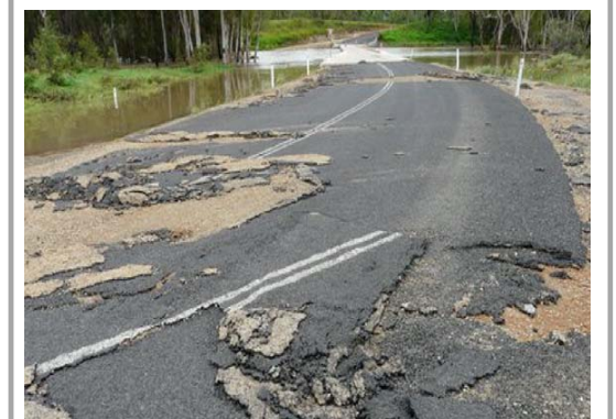
Above: damage to the Mitchell River Crossing on Strathleven Road at Gamboola, a Tablelands Regional Council betterment project
