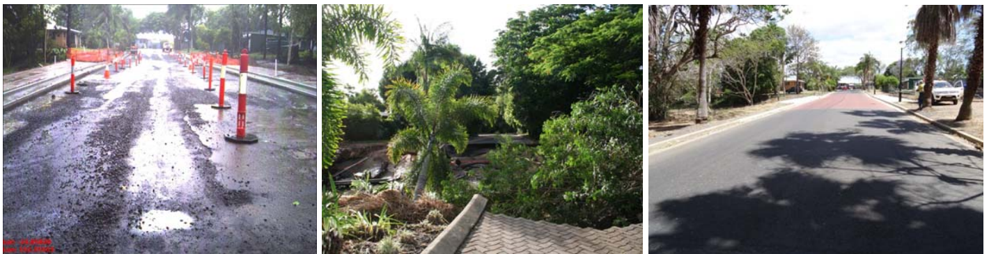
Damage (left and centre) and works following completion (right) on Mariners Way, Bundaberg
