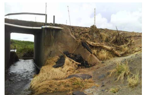
Debris build-up and scouring of the approaches.
