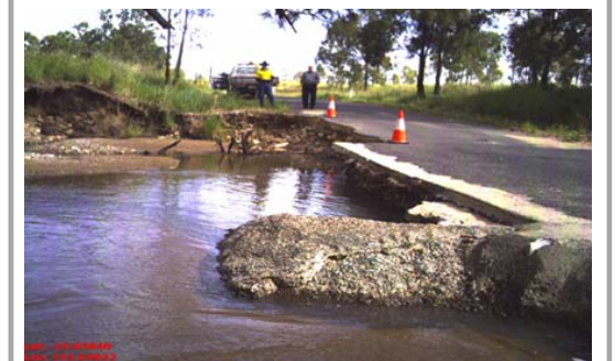
Above: damage to Gaeta Road (top) and Wonbah Road (above), Bundaberg Regional Council
