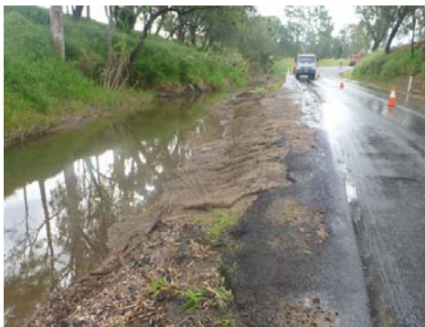
Left: damage to Woodlands Road, including scouring of the road shoulder and pavement rutting
