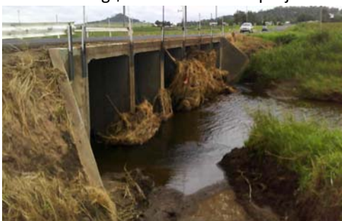
Debris build-up impacting culvert flow-through.
