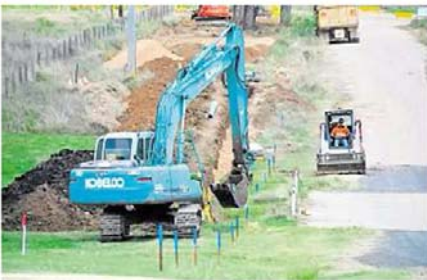
NEW SUPPLY: Gayndah's town water will be sourced from above Claude Wharton weir. PHOTO: BRANDON LIVESAY
