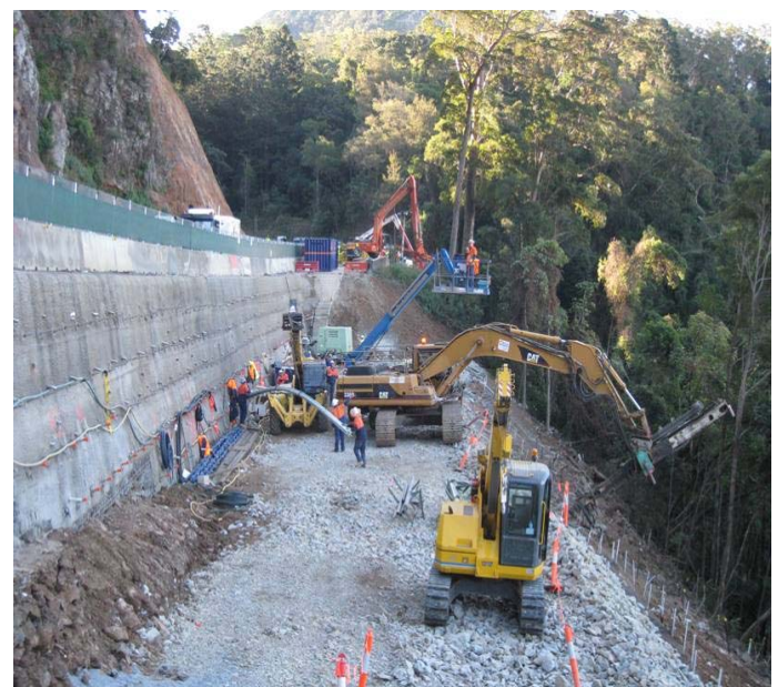
July 2011 Reconstruction works: Slope stabilisation work at Cunningham's Gap west of Claytons Gully, temporary soil nails on left, permanent nails in progress on right.
