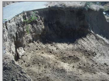
Above: Broadmere Road, Taroom was badly damaged by floodwaters in January 2011
