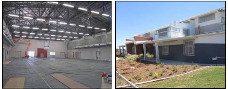
Above: Updated progress of Cyclone Shelter - Bowen SHS - nearing completion in mid October
