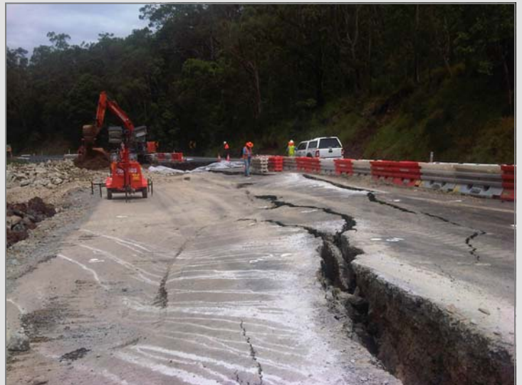
Above: damage to Cunningham Highway, Cunninghams Gap
