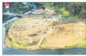
PHOTO BY PETER ROYLE: Aerial view of Colleges Crossing being reconstructed. August 2012.
