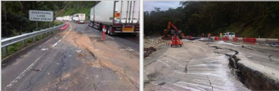
Above: Damage to Cunninghams Gap
