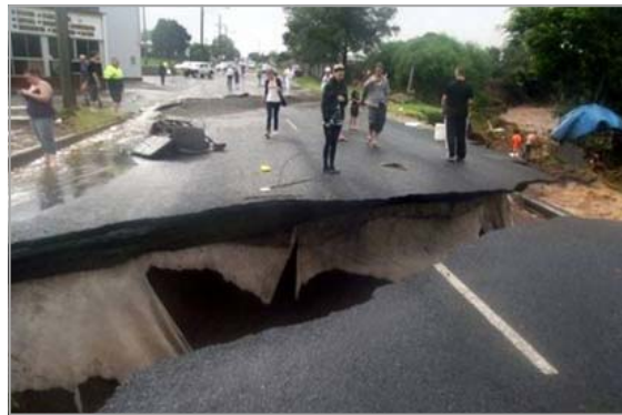
January 2011 flash flood damage
