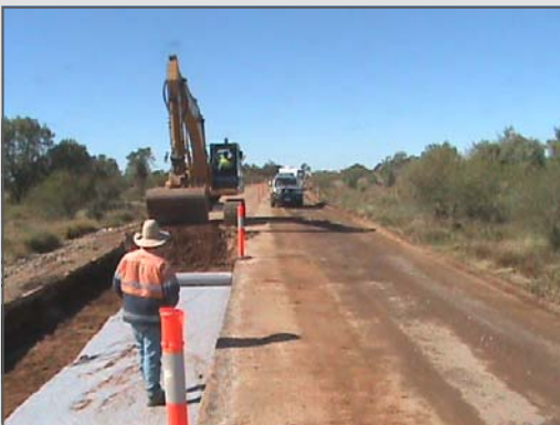
Above: Construction - placing geofabric as a foundation at the Rutchillo Creek Floodway on the Landsborough Highway
