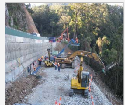
Slope stabilisation at Cunninghams Gap, west of Clayton Gully (temporary soil nails on left, permanent nails in progress on right).
