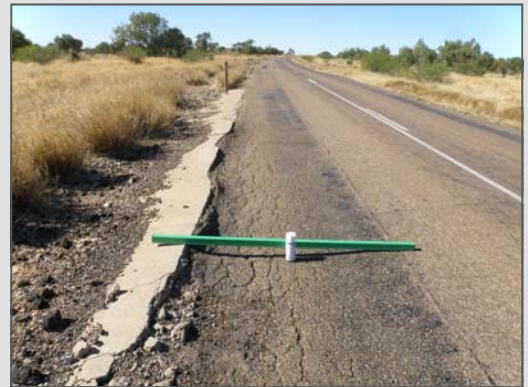
Above: Preconstruction - 2011 flood event damage at Rutchillo Creek Floodway between Cloncurry and McKinlay (Landsborough Highway)
