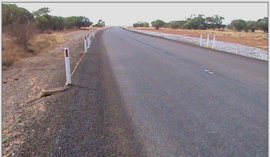
Above: Post construction- Rutchillo Creek Floodway, prior to line marking and showing rock mattresses.
