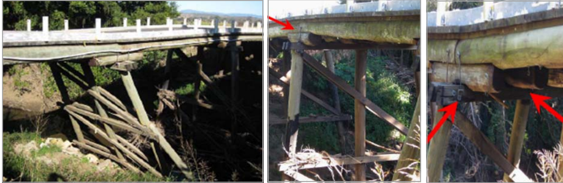
Stokes Bridge damage
