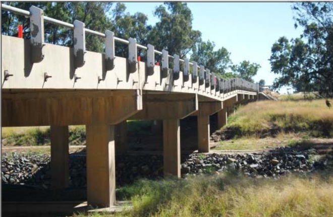
Above: June 2012 - Pier 5 dropped more than 40 cm
