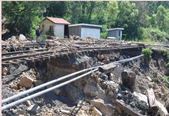
Rail line from Brisbane to Toowoomba destroyed – Spring Bluff, 19 January 2011. Source: Toowoomba Chronicle
