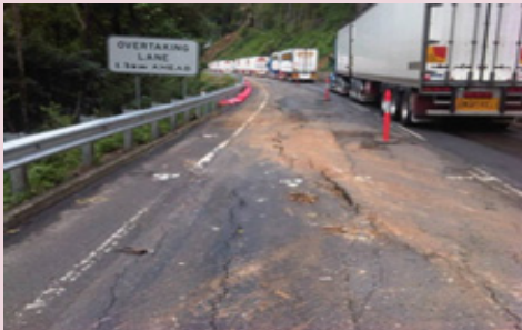
Damage to Cunningham's Gap
