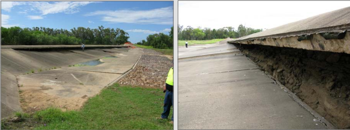
Above left and right: Moolabah Weir after extensive flood damage
