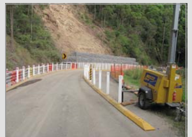
Above: Interception wall constructed as part of emergency repairs at Hairpin Bend.
