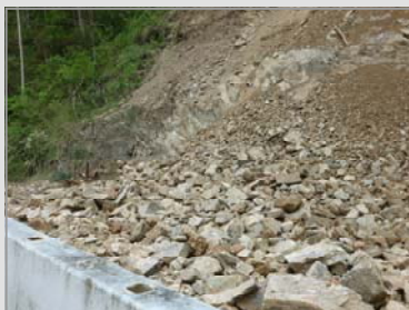
Above: Landslip damage to the uphill embankment, Samford-Mount Glorious Rd at the site known locally as the Hairpin
