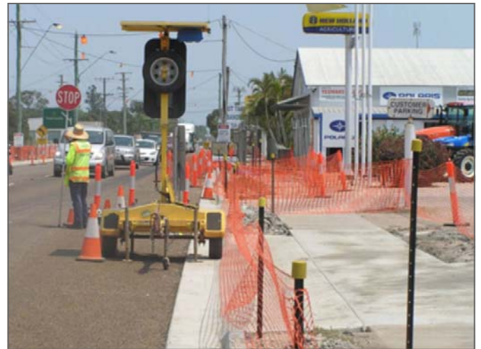
Case study: Reconstruction work on the Bruce Highway through the centre of Brandon, approximately 85 kilometres south of Townsville.
