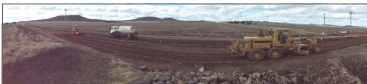
Case study: Toowoomba Regional Council uses local materials to rebuild Evanslea Road.
