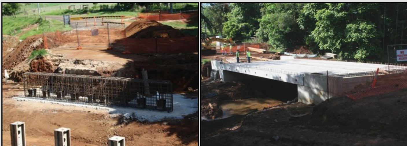
Reconstruction works in progress on Figtree Close Bridge undertaken by Tablelands Regional Council (Images taken 14 December 2011)
