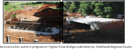
Reconstruction works in progress on Figtree Close Bridge undertaken by Tablelands Regional Council
